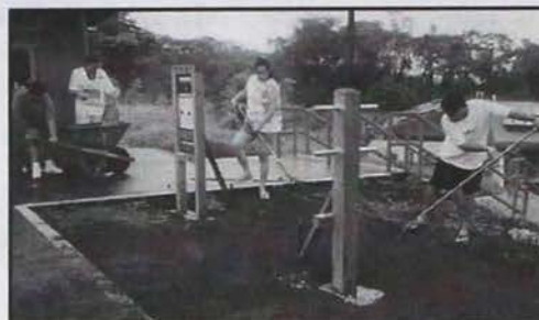
Hawaii-Hilo members worked to improve the Hilo Campus environment by helping build one of the exercise field stations at the Athletic Department.
